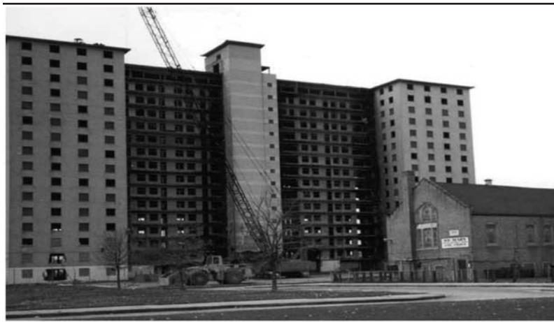
Figure 2: Photograph of Robert Taylor Homes Located at 48th and State Streets With Wrecking Crane
