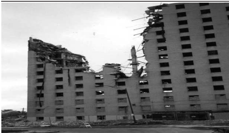
Figure 4: Photograph of Demolition of Robert Taylor Homes Located at 41st and Federal Streets
