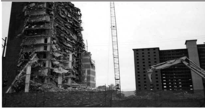
Figure 3: Photograph of Demolition of Robert Taylor Homes Located at 48th and Federal Streets
